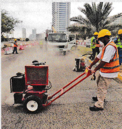
Routing cracks prior to sealing creates a reservoir that improves the adhesion of cracksealing material.
