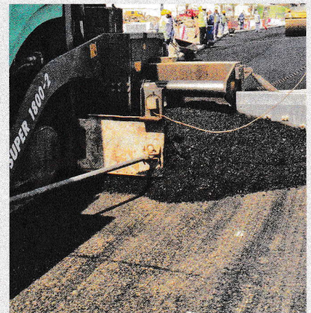
Proper sealing of cracks in a milled surface will help prevent the cracks from reflecting up through the new overlay.
