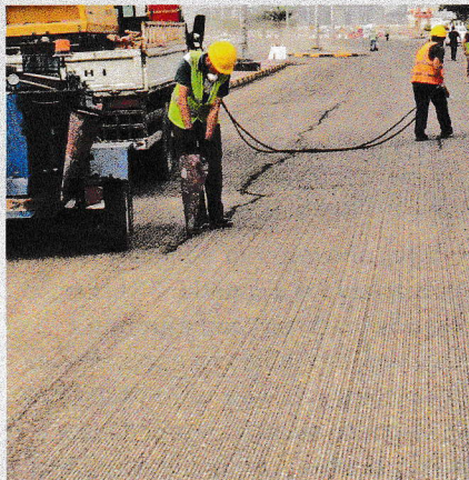
Material can be gravity fed using cones into the crack area – a simple, fast, low-cost, and easy method to carry out.
