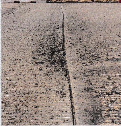
It's essential to thoroughly clean routed cracks of any debris as leaving any loose material or dust in place can result in a failure of the whole process.
